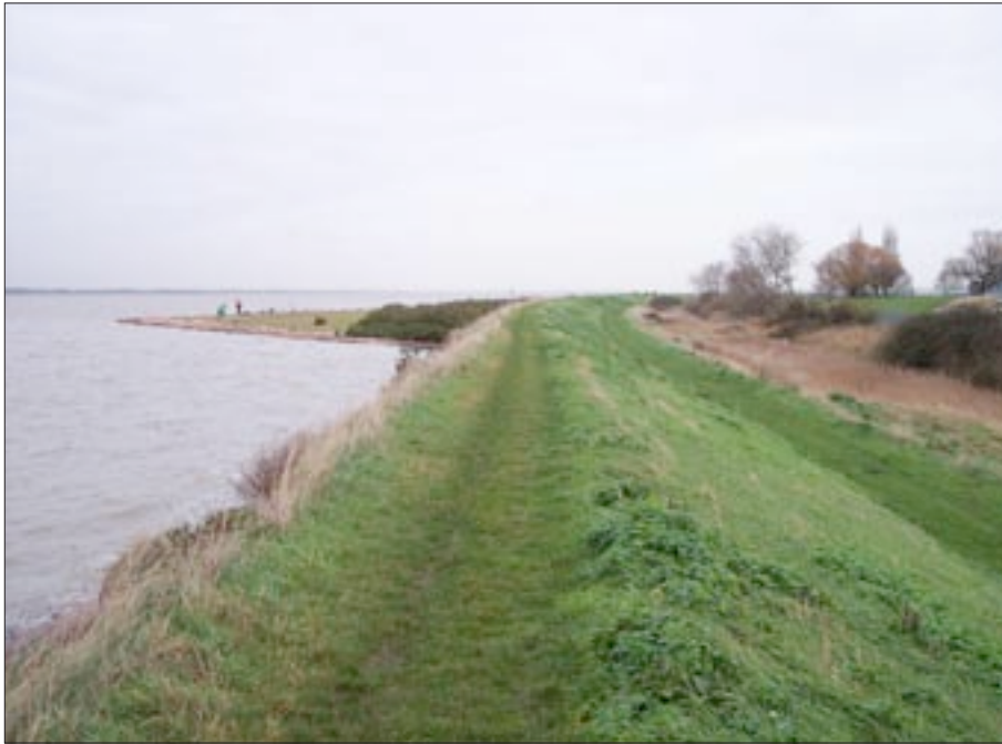
Photo 6. Considerable topographic differences either side of the embankment significantly increases the vulnerability of the power station to flooding from future climate change.
