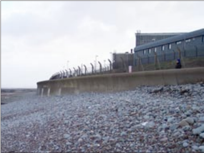
Photos 3 and 4. Extensive gabions and seawall comprise the defence structure for the power station. Increases in storm surge heights and frequency of storm events could undermine the integrity of this system and result in inundation at the site.
